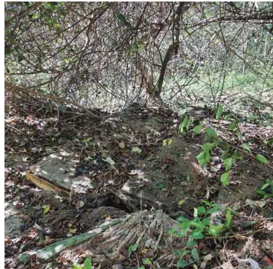
Fig 2c. The manholes on the pipeline remain open for the time being.
