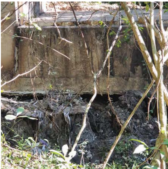
Fig. 2b. Some areas of the pipeline have been undercut and will need to be repaired.
